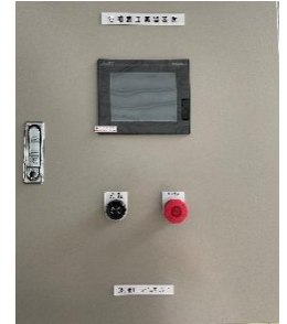
Touch panel control cabinet
